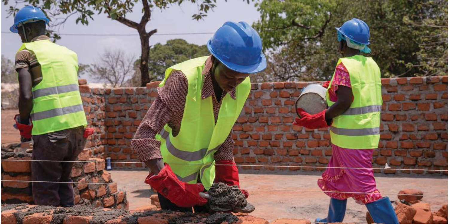
© UNHCR/Esther Ruth Mbabazi. South Sudanese refugee working in construction at the Bidibidi settlement in Uganda.
