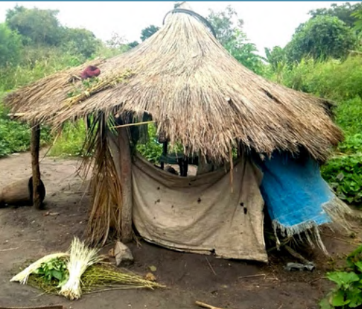
One of the tukuls before reparation. Photo: JRS.
