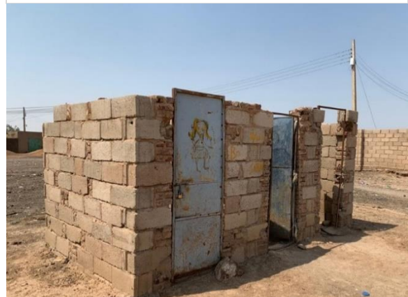
Only communal latrine in Dar Es Salaam Block 7
