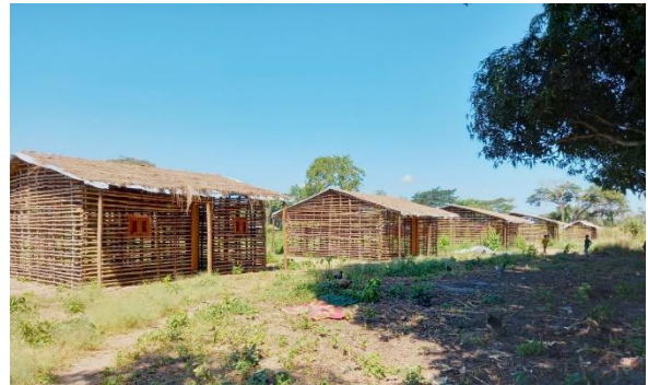
Ongoing construction of shelters by UNHCR and partner SI in Mueda District, Cabo Delgado. ©UNHCR/ Nilton Mungamba
