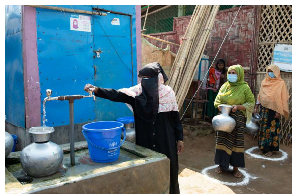
Bangladesh. New treatment plant in Kutupalong camp provides fresh water for refugees @UNHCR/ Kamrul Hasan
