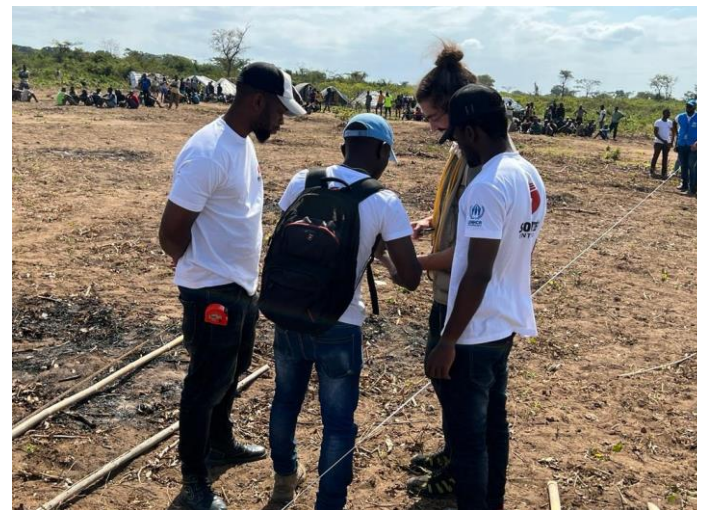
Site preparation to set-up reception facilities in Lyanda IDP site, Mueda ©UNHCR/Gure Abdi
