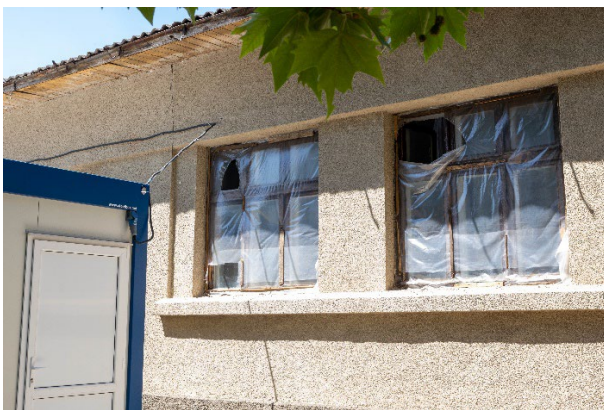
Damaged windows at a rural RAC
