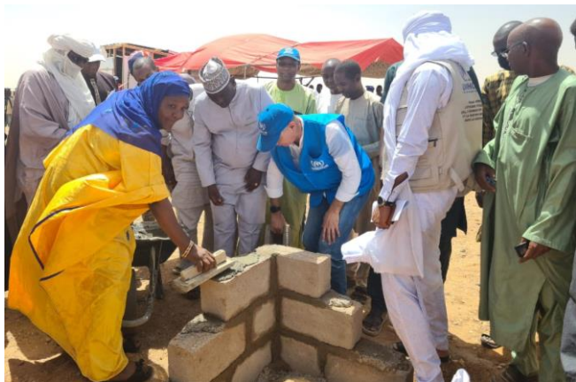
UNHCR launched the construction of two buildings with three classrooms, an office and a store in the Mai Adoua school compound, in Agadez. UNHCR/ Amadou Maman Guimba
