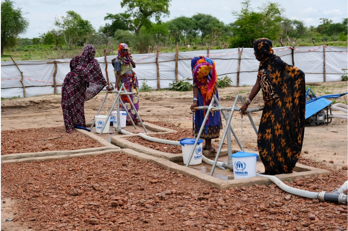
In the Central African Republic, refugees from Sudan have been relocated to the Korsi site in Birao, where construction works for family and community shelters are ongoing. They are provided with multisectoral assistance, including water, food and CRIs. © UNHCR/Josselin Brémaud
