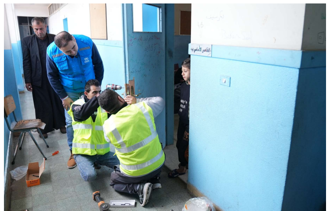
UNHCR provides partitioning and other shelter rehabilitation for displaced families in collective shelters in the North. ©UNHCR/Houssam Hariri
