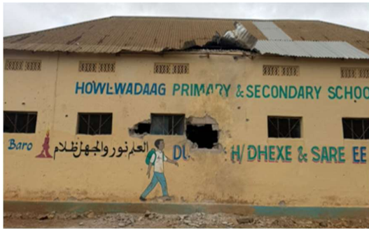
Figure 1: Howlwadag School damaged by gunfire
