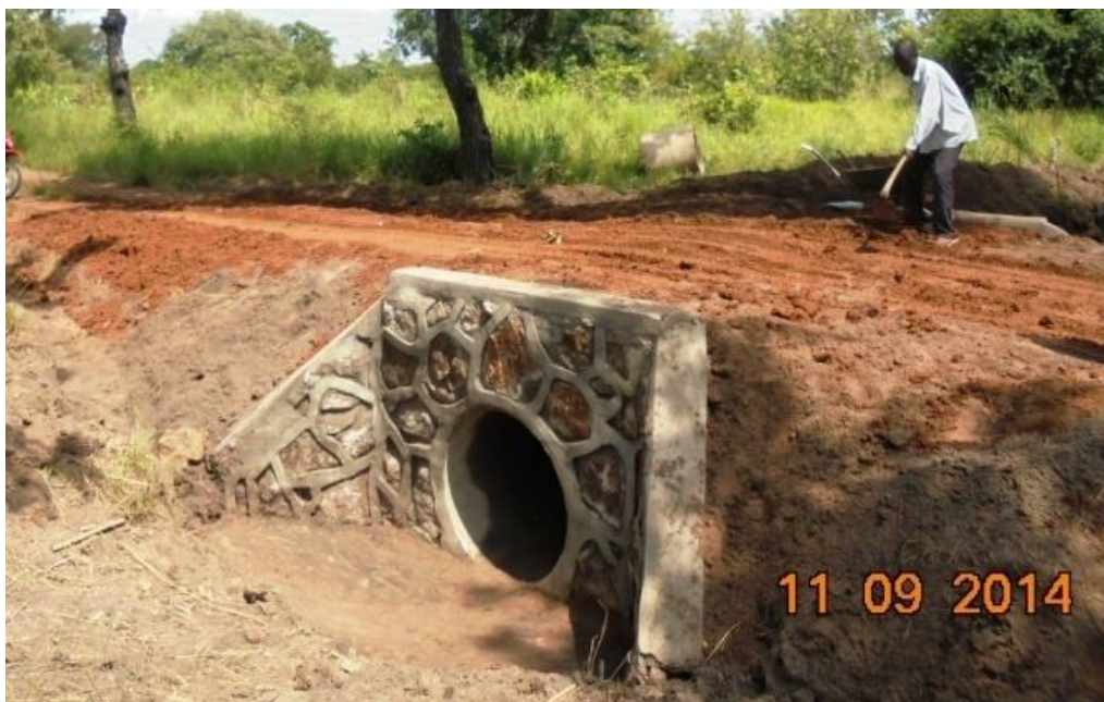
Completed head wall pending further road works along Simbili- Ariwa road. ©DRC-DDG/Patrick
