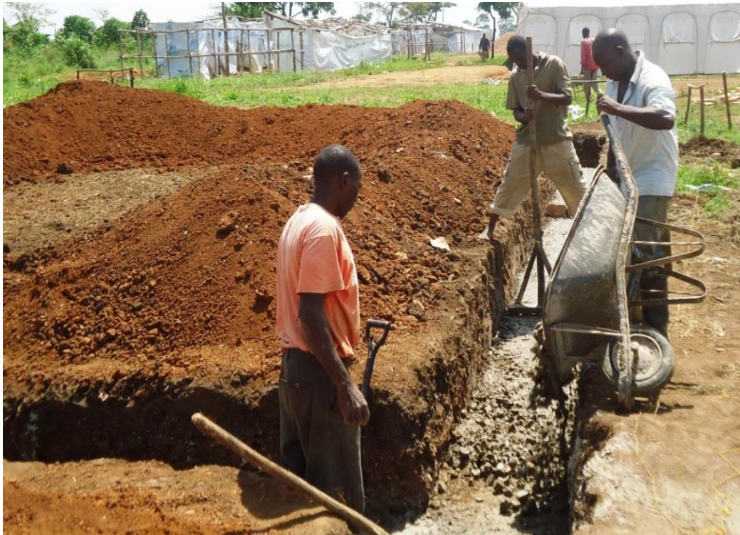
Construction work of a reception centre at Kagoma is underway in Kyangwali settlement. ©UNHCR/J.K. Lotweny
