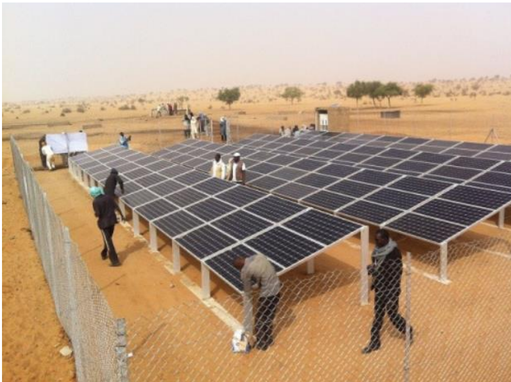
Solar energy system in Eukinawane for the provision of drinking water. The system serves populations in the refugee hosting area of Intikane, as well as the local population. © UNHCR/Boubacar Siddo
