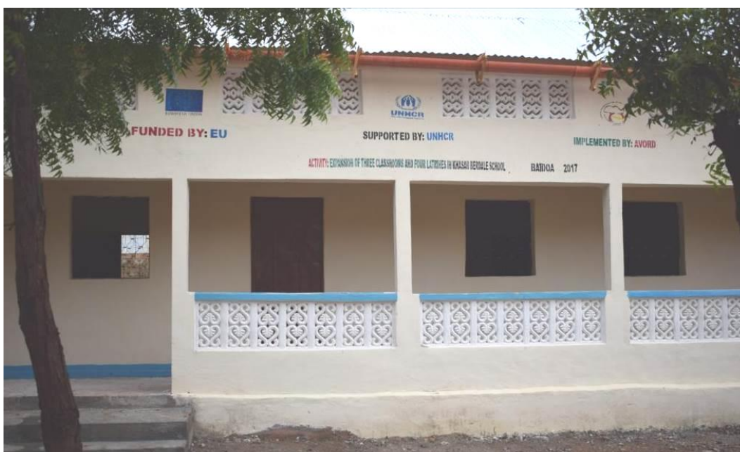
Ongoing extension of a primary school Khasab Berdale School (four classrooms and four latrines) in Baidoa. In 2017, UNHCR has already rehabilitated eight schools and continued with rehabilitation of two schools. © AVORD / Baidoa, October 2017
