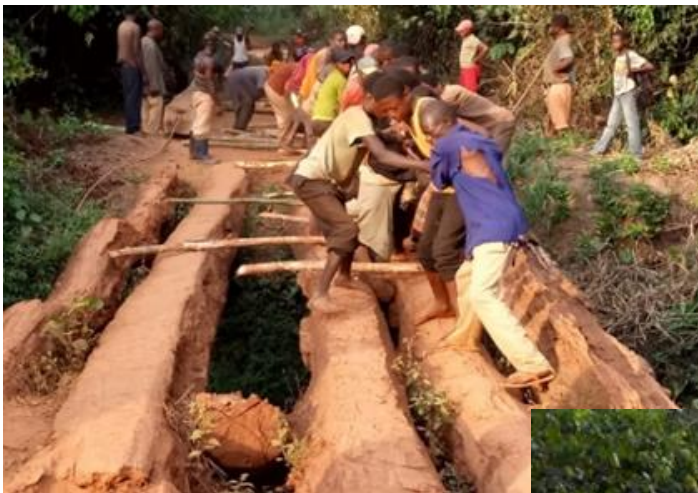
Rehabilitation of a bridge along the road between Monga and Ndu, Bondo Territory, Bas –Uele Province © UNHCR/G. Nentobo
