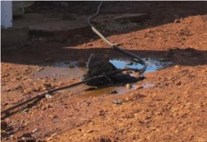
Figure 7: Leaky water-distribution pipe in Bouday B
