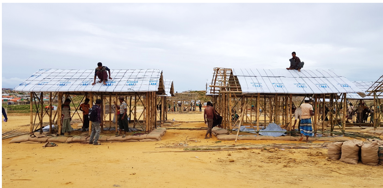
Workers constructing shelters in Camp 4 Extension, the new land allocated by the government and leveled by UNHCR and partners as part of the SMEP project. © UNHCR/Dalal Alsharhan
