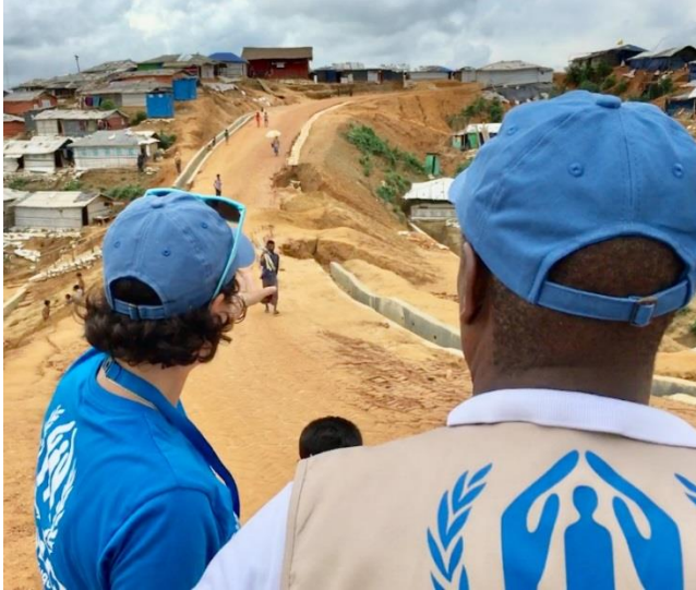
UNHCR's Representative in Bangladesh examining the monsoon response in Cox's Bazar. Roads affected by the heavy rain being repaired by SMEP, a joint UNHCR/WFP/IOM engineering project, and Bangladesh Armv. Photo: ©UNHCR/S. O'Brien
