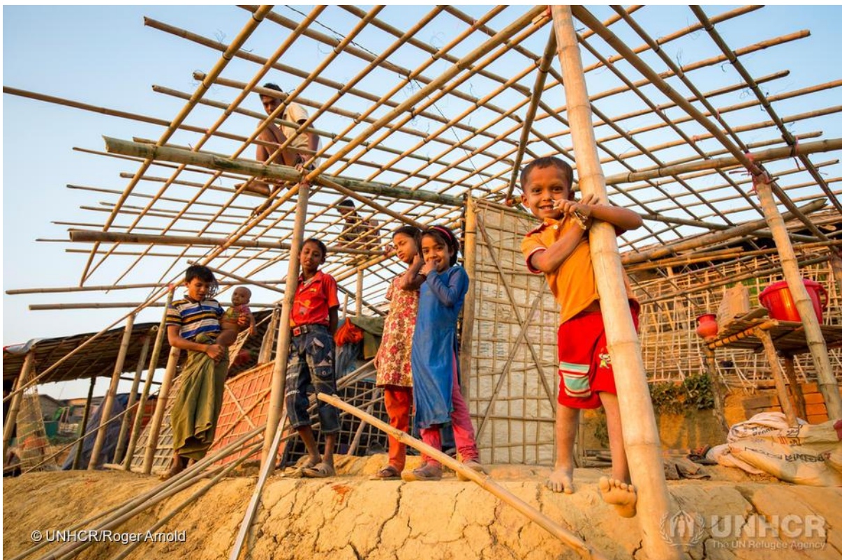
Rohingya refugee families prepare for the monsoon by building new reinforced shelters with materials supplied by UNHCR. © UNHCR/ Roger Arnold
