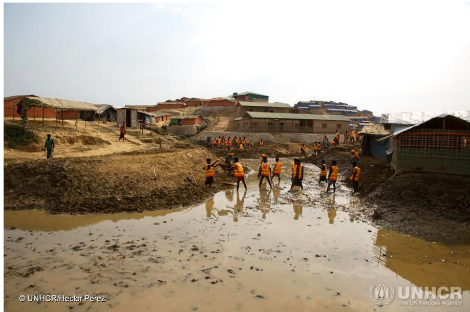
UNHCR is undertaking monsoon preparedness, including essential infrastructure work such as the widening of canals and gullies, digging culverts, flattening land, and relocating families to safer places where new land is available. © UNHCR/Hector Perez
