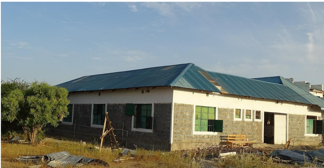
Construction of the Dhobley General Hospital which will be available to around 72,000 persons. © UNHCR/2019
