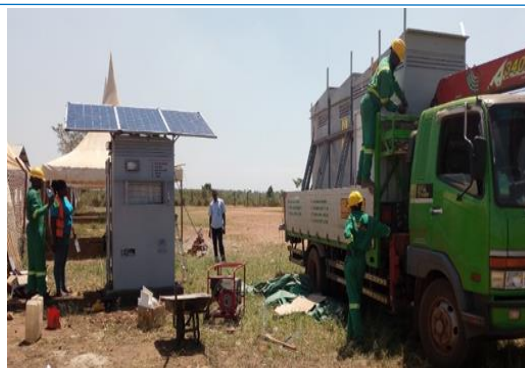
Installation of a Solar Powered phone charging Kiosk in Magamaga G, Kiryandongo. Photo©Katuura P. UNHCR
