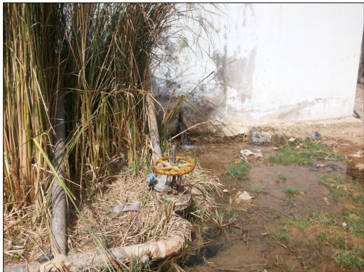
Figure 1: Leakages from a storage facility
