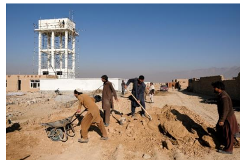
Returnees build a water tower to supply fresh water to their community as part of cash-for-work initiatives under UNHCR's community-based protection programme. © UNHCR
