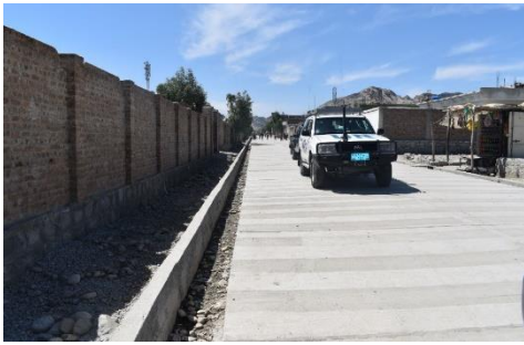
UNHCR encourages other partners to engage in projects to support returnees and host communities. UN-Habitat constructed this road in Daman. © UNHCR
