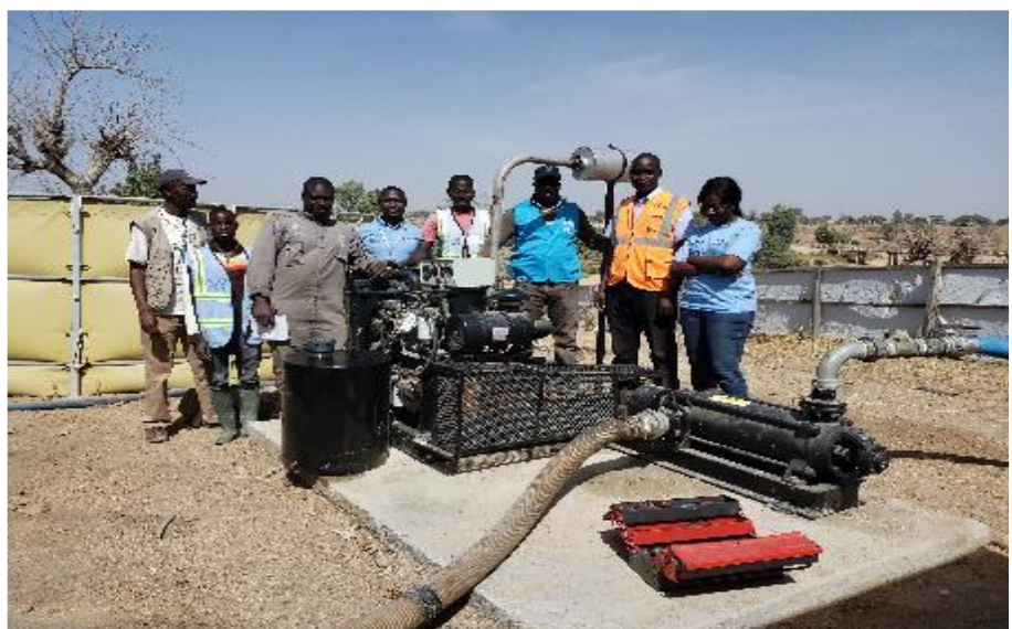
Technicians fixing the new high- pressure water pump for Mokolo-Minawao water supply network - UNHCR @ Djarmatna Kadessou
