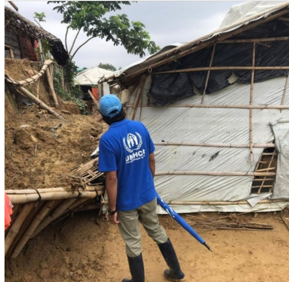
UNHCR staff examining a broken retaining wall that collapsed under heavy rain. Photo: © UNHCR/O. Sanchez Pineiro
