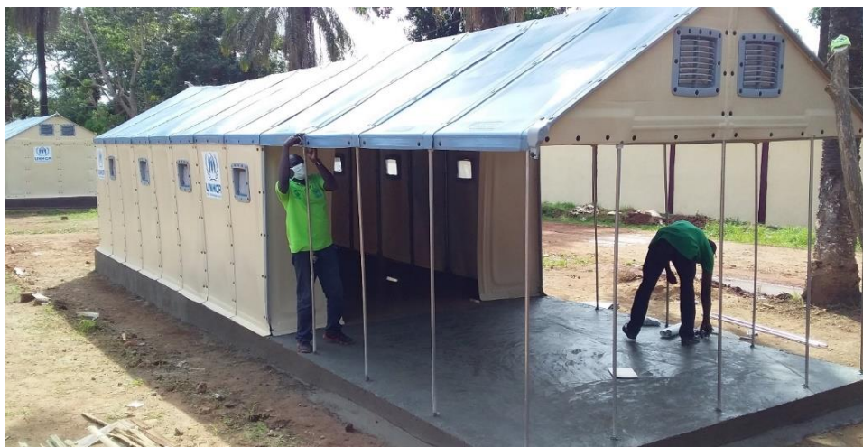
Installation of RHUs by UNHCR's partner AIRD at the University Hospital of Bambari. ©UNHCR CAR
