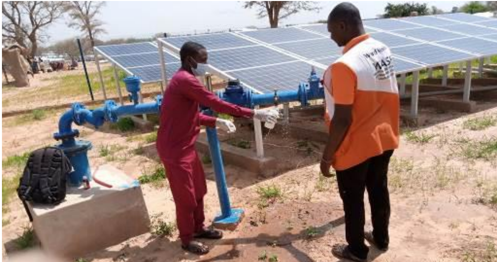
Engineers verifying the quality of water at the water pumping station of Dan Dadji Makaou © / UNHCR.
