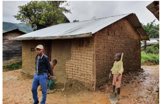
An internally displaced family in the territory of Walungu is building a transitional shelter. © UNHCR / Duga Amani
