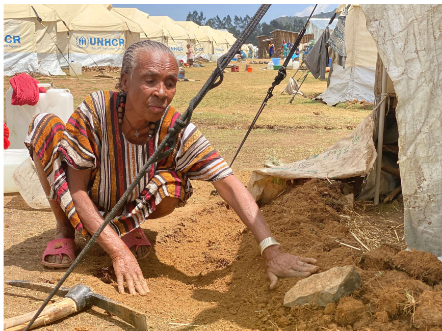
Gebre is digging a trench to redirect rainwater from flooding her home in Kulichmeda IDP site (Amhara). ©UNHCR/D. Dieguen, February 2021
