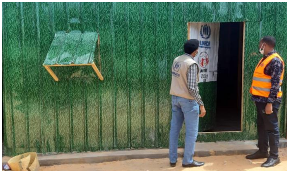
UNHCR staff checking one of newly constructed 60 shelters ready for handover in Kismayo. © UNHCR
