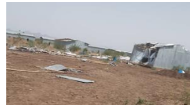
Damaged communal shelter in Boredde Gelede-Lemi IDP site due to heavy rain © Dawit Daricha UNHCR
