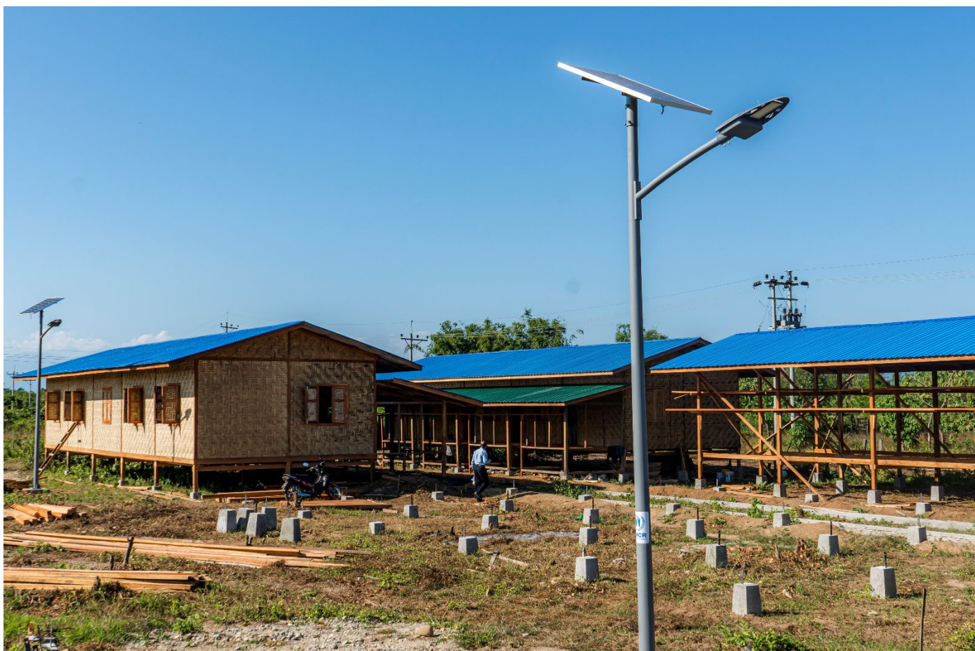
UNHCR provides targeted shelter support to IDPs in Kachin State. New homes are constructed for families and solar streetlights are installed to illuminate pathways and provide a sense of security. © UNHCR/Hkun Ring
